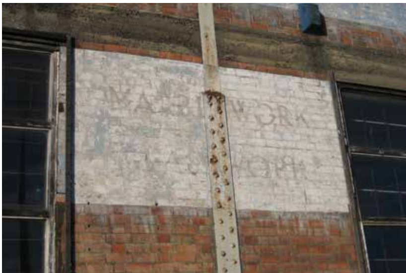
Detail of some of the lettering on the eastern side of the building: 'Marblework' and 'Glasswork'
