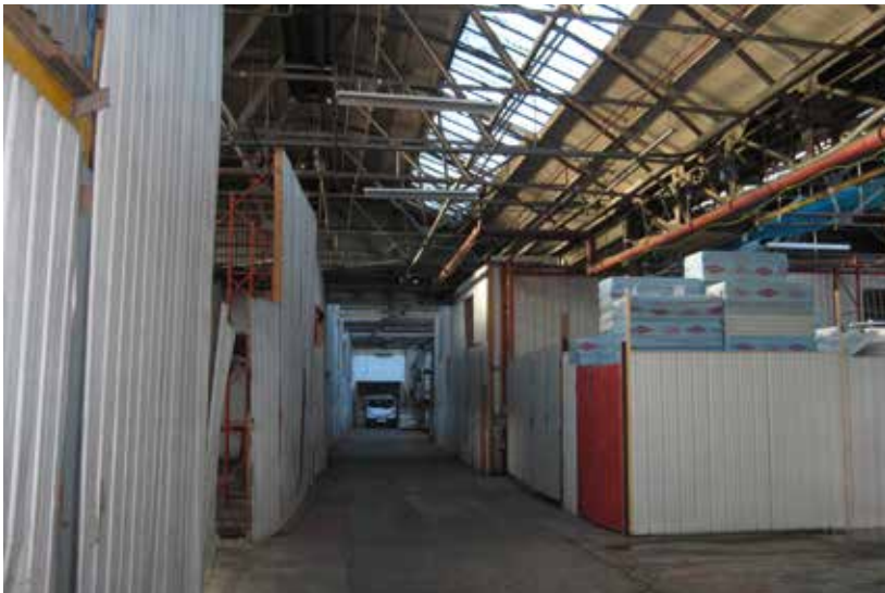
One of the bowstring truss roofs with inserted storage units and offices beneath
