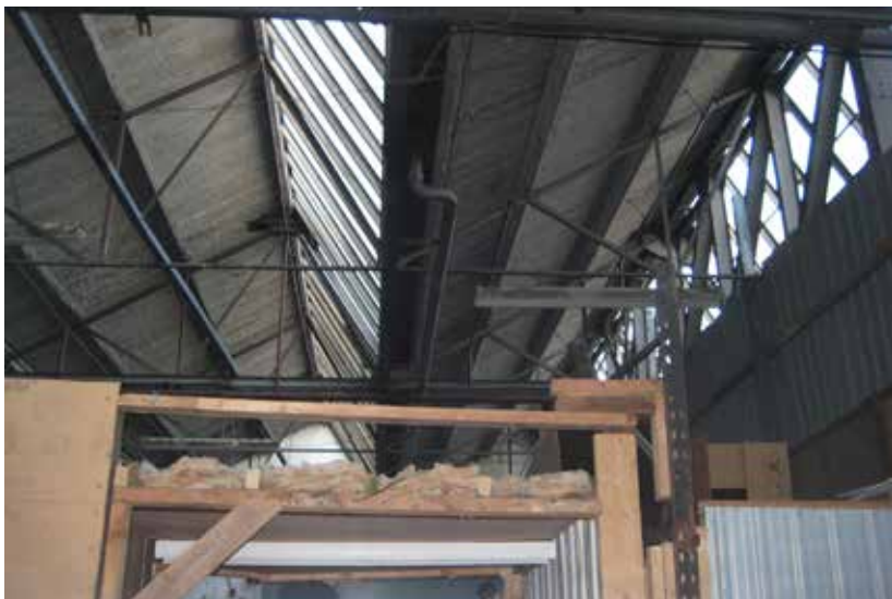
View inside the northlight building over the tops of the inserted storage units and lock-ups
