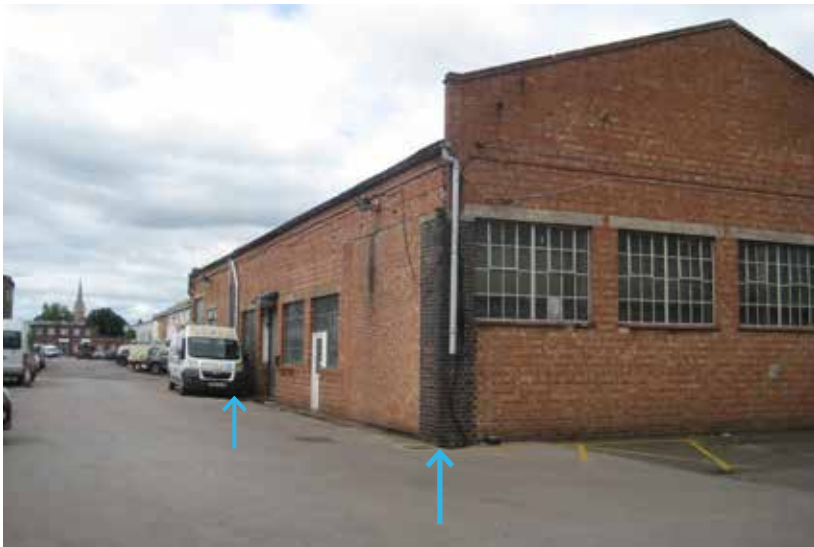
View south-westwards along the south-eastern elevation of Unit 1; the space between the two dark brick piers (marked) was historically openable, but has been infilled with brick
